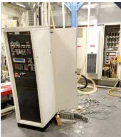
Old control cabinet
