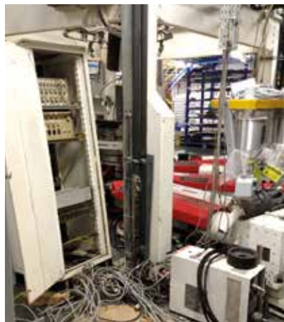
Old control cabinet "separated"
