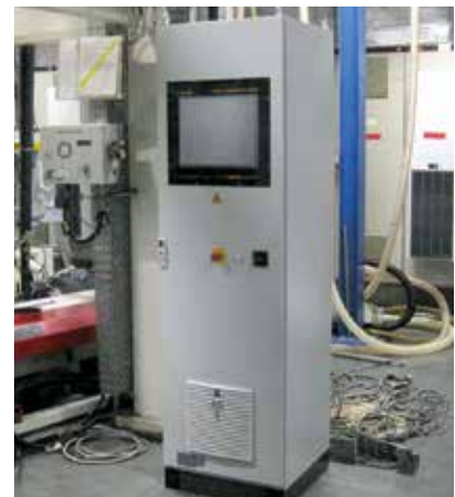
New control cabinet ready for use
